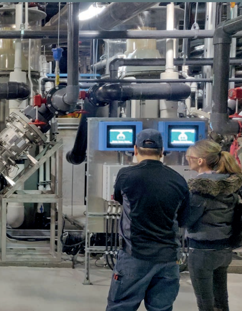
Installation of the Atlantium UV systems in a RAS facility in N. America for Myxobolus Cerebralis and Myxosporean protection. Photo: ©Atlantium
